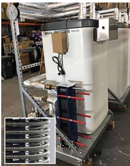
Heat exchange in DHW plumbing using PHX and stainless steel coils.
